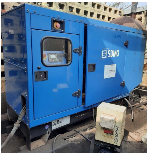
Diesel generator that provides power supply on the Customer's facility (GSM mast)
