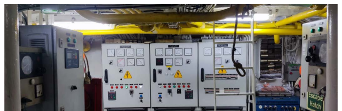
Generators and power management control panel
