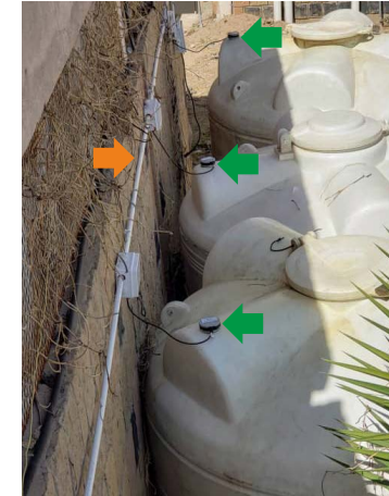
DUT-E 2Bio sensors (➡) and S6 cable system (➡)
