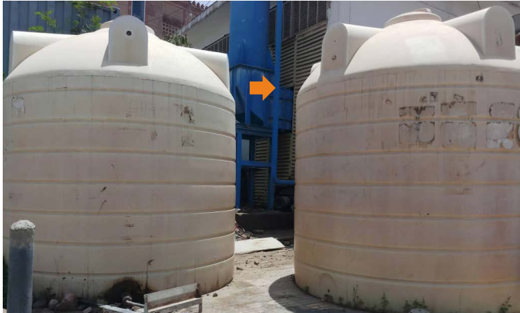
Tanks supply fuel to generators (➡)
