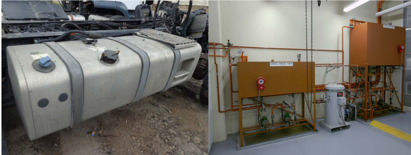
The fuel tank of a truck (left) and fuel storage tanks for diesel generators (right)
