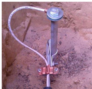
Figure 11 – Example of grounding the Station power supply generator using a metal rod
