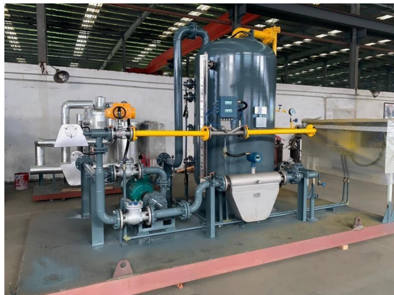
Figure 23 — Example of an LC Corio liquid counter installed in a pipeline at an industrial facility
