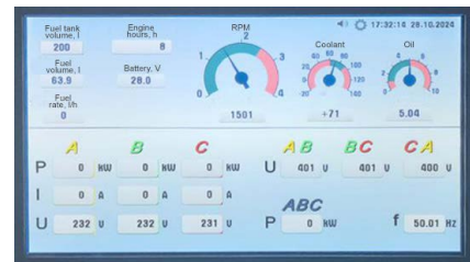
Fuel and engine data is displayed on the operator's panel.
