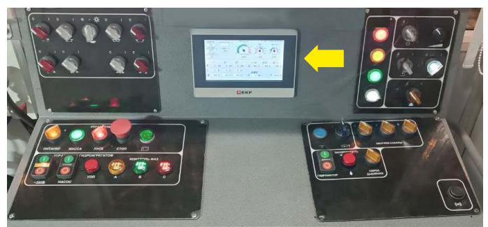
Generator operation data is shown on operator's panel
