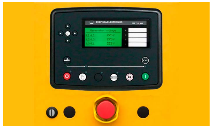
DSE 7320 MKII controller installed on the generator
